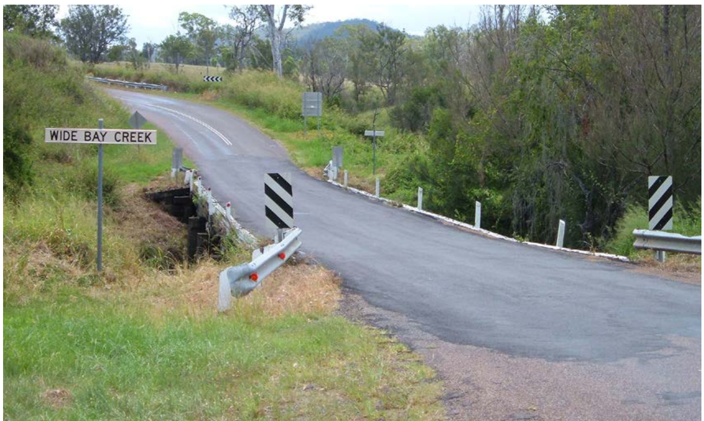
Wide Bay Creek bridge before replacement under the Regional Bridge Replacement Program
